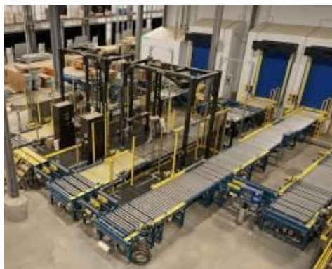
Chain Conveyor in a Cold Storage
