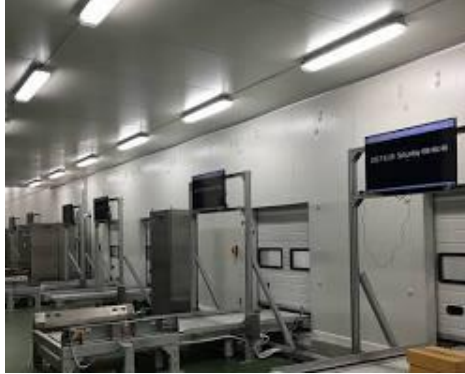
Roller Conveyor in a Cold Storage
